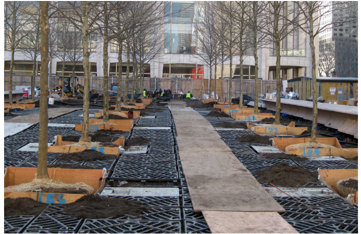
Soil cell installation at Lincoln Center New York (Source: DeepRoot on Flickr.com)
