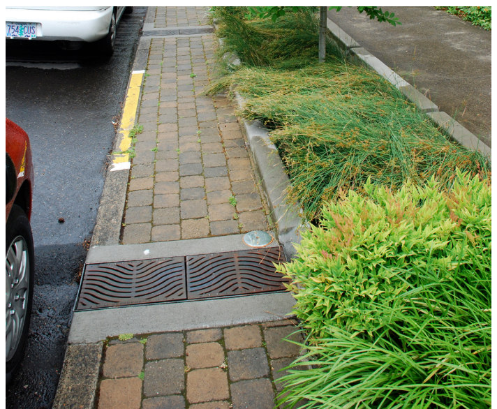
Bioretention planters for stormwater management, Portland OR
