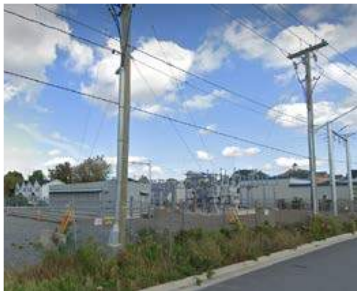
Aberdeen Street Substation
